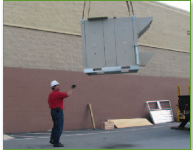
Crew lifts the Rooftop Systems' ERV into place during the initial installation at the Target Store in Philadelphia.
